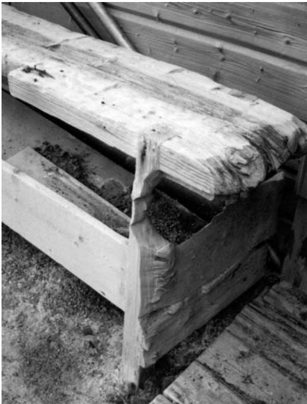
Fig. 6. Severely weathered end carpenter's work bench. January 1990.
