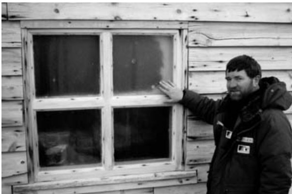
Fig. 13. Abraded glass of window on southeast wall, Scott's hut Cape Evans. January 1998.
