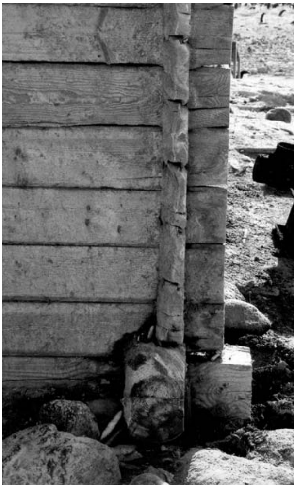
Fig. 4. Weathered northeast corner, Borchgrevink's 'stores hut' with coating of salt and sand particles. January 2003.
